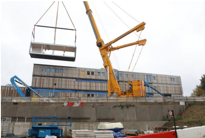
Image of module cabins to form the replacement site accommodation block for Euston Station works and the new Construction Skills Centre
